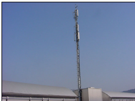
figure 12-14: View of the BEGF installation
