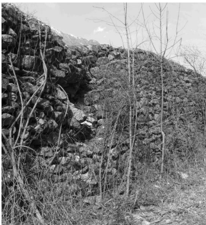
Figure 4 This 3-m-tall gabion embankment was cleared by a block after an impact more than 1 m below its crest, by a block having an upward incident trajectory (Ste Marie de Cuines (73), France).(S. Lambert)
