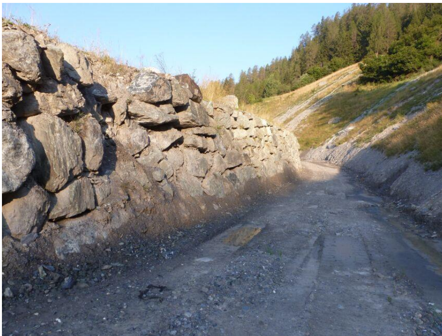
Figure 11 Damage of a RPE with rockery at the uphill side after block impact (Tiefbauamt Graubünden)
